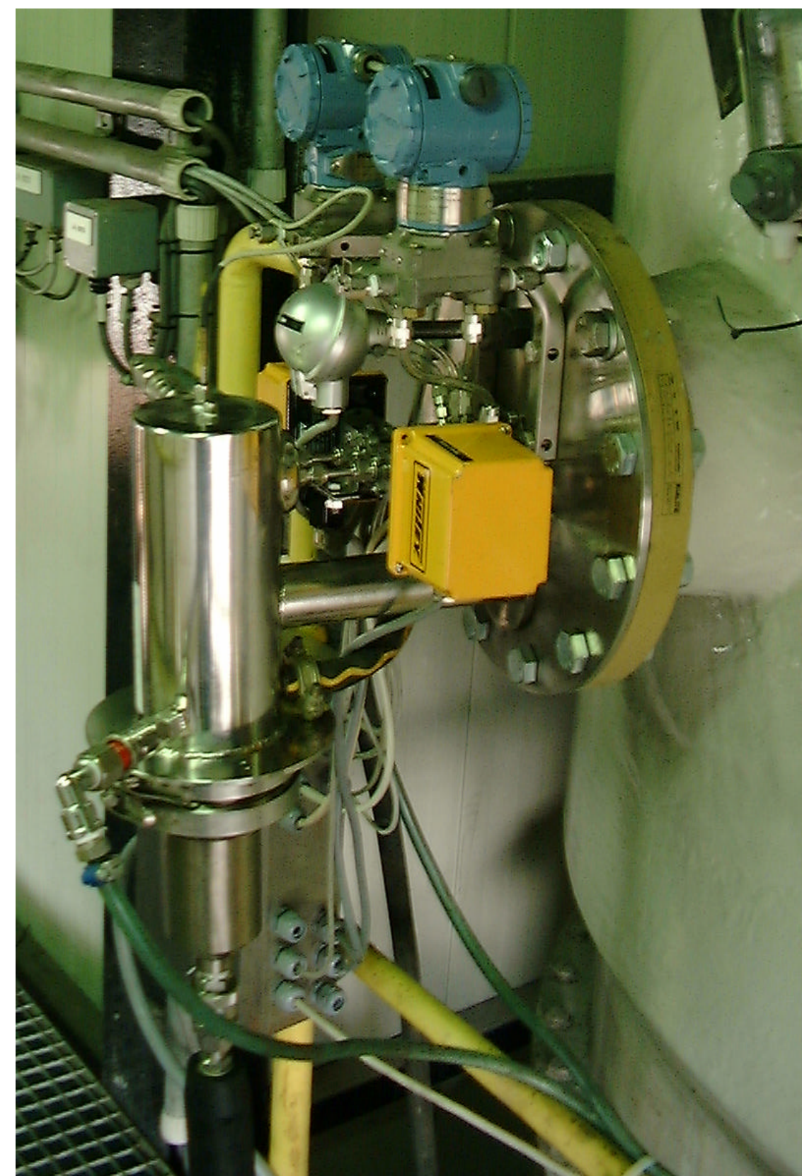
Picture 2: sampling unit installed at the hazardous waste incinerator
